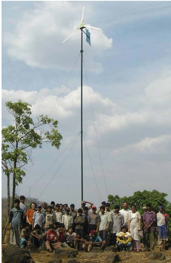
Here is an example of the wind turbine that will be built in Rwanda. This was constructed in rural India, under the direction of Dr. Mark Pitterle and Rachel Werther with CU Denver. Dr. Pitterle will be one of the engineers traveling to Rwanda for the Wind Turbine Workshop.
